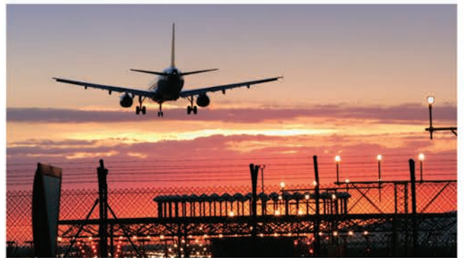
Airfield Ground Lighting Cables
